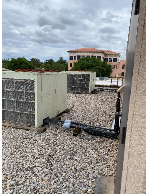
Figure 12 - Back-up DX units on the roof of the Computer Center building.
