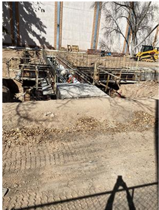
Figure 18 - Branson Library Open Tunnel; under repair
