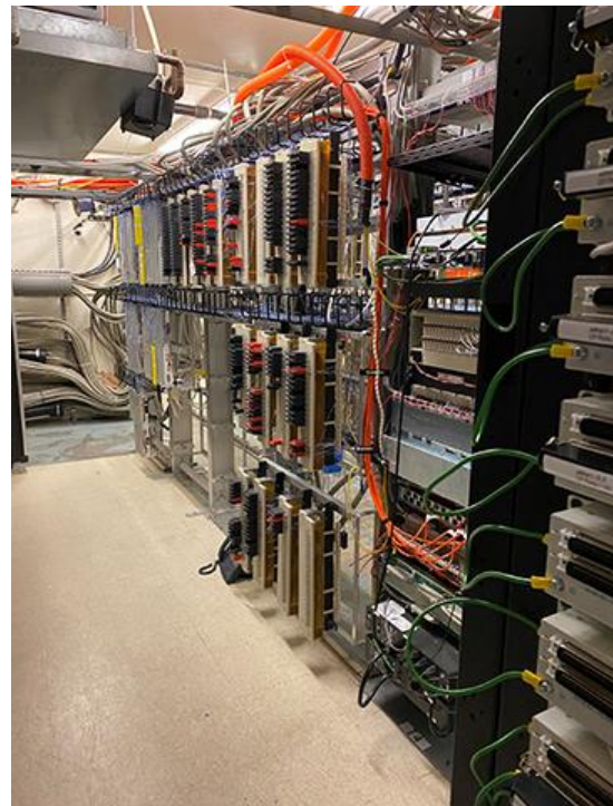
Figure 3 - Copper cabling; infrastructure distribution fused protectors /active Century Link (lumen) rack
