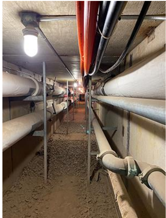
Figure 16 - Science Hall Tunnel; Building #391 – This picture represents new innerduct pathways
