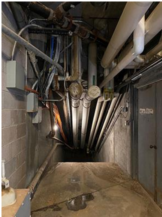
Figure 17 - Tunnel to Building 126 – This picture represents existing and newly installed innerduct pathways for optical fiber cable.
