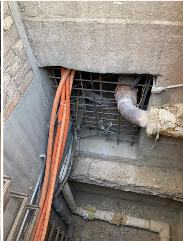
Figure 20 – Exposed innerduct pathway
