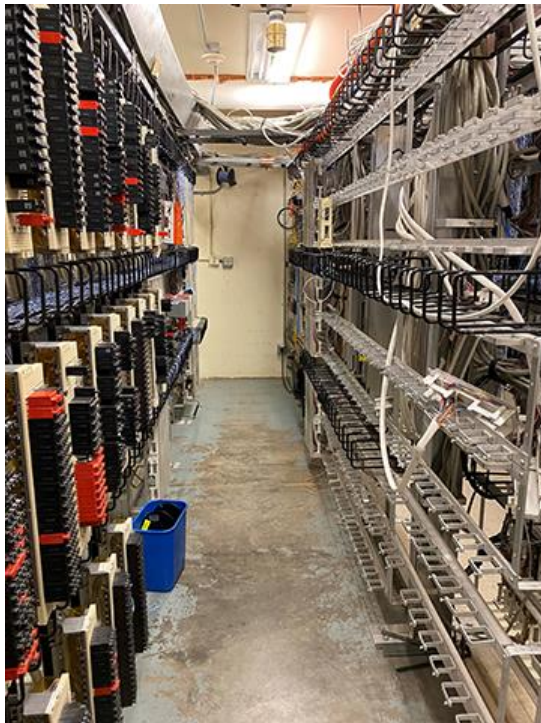
Figure 2 - Milton Hall Infrastructure racks – distributing 12,000 pairs of copper throughout the campus
