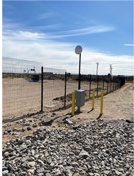
Figure 23 - Communications of the solar farm are being handled via microwave.
