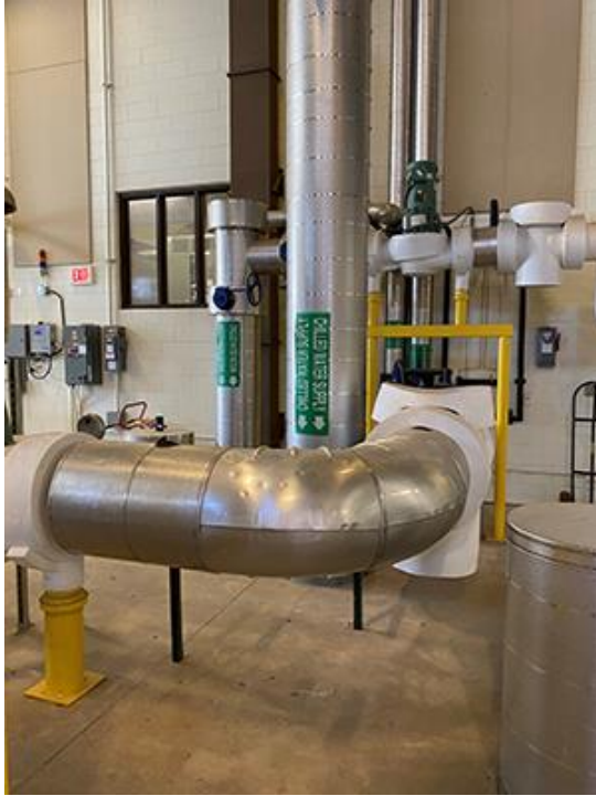
Figure 22 - Pictured; inside the chilled water plant
