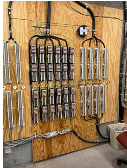
Figure 27 - Building #126 (Computer Center) entranced facility cross-connect field in basement
