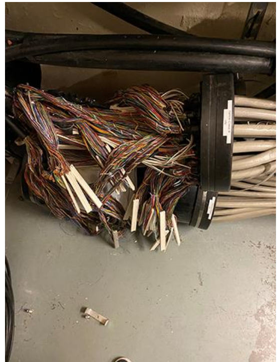
Figure 5 - 710 splicing of copper infrastructure distribution splicing
