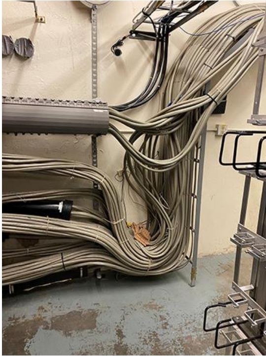
Figure 2 - Transitioned cabling from OSP to indoor riser cable, terminated on Homoco distribution frames (racks)
