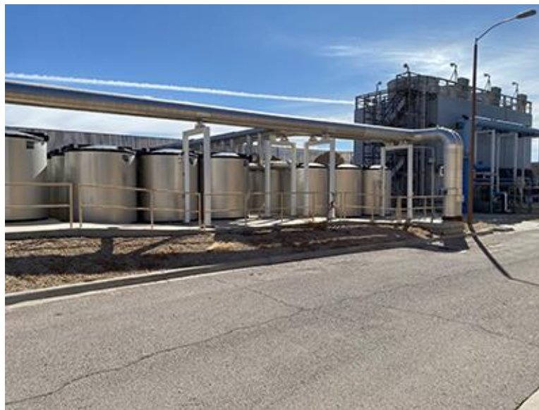
Figure 24 - Ice storage farm located outside of the chiller plant.
