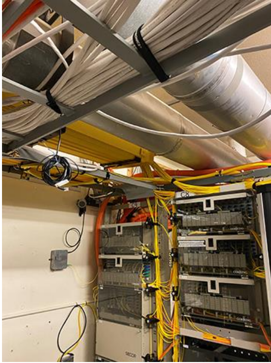
Figure 8 - Optical fiber campus distribution racks with roof drains installed directly above the racks.
