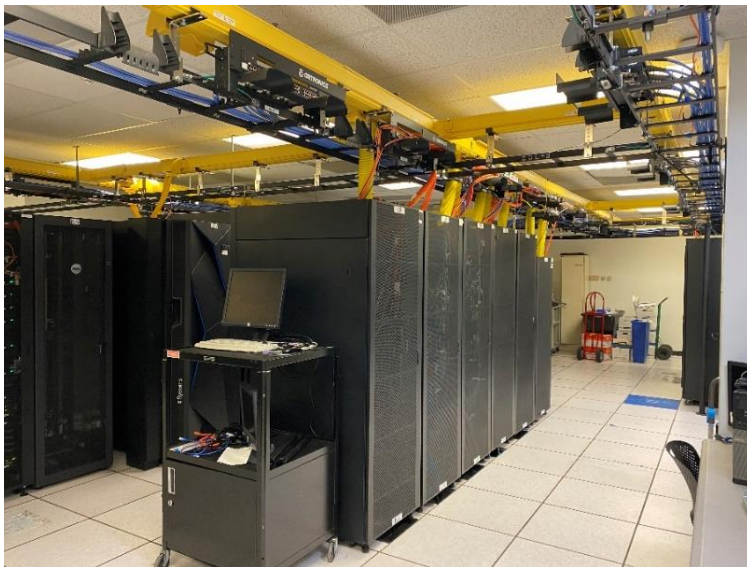
Figure 10 - Main Data Center Space
