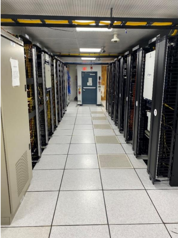
Figure 11 - Network Operations room.
