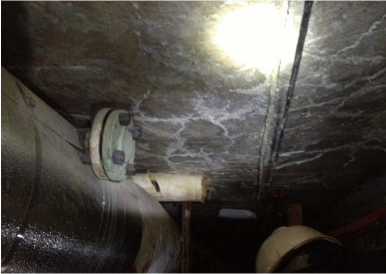
Lid Section Failure
